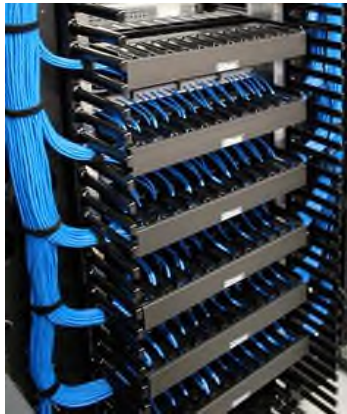
Good example of cable management
