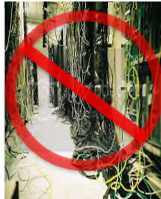
Bad example of cable management
